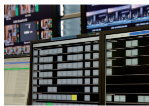
Central alarm system
