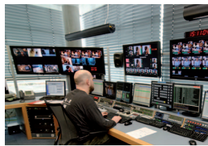
Master control room
