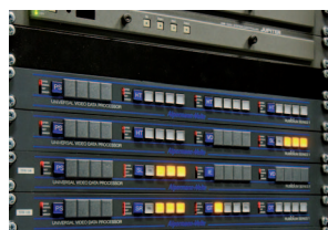
Time control system
